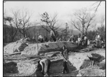
CCC workers building the Great Lodge at Douthat State Park, Courtesy of the Library of Virginia
